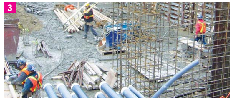
January 12, 2007 No winter hibernation on the work site—the foundations and basements of the new buildings take shape.
